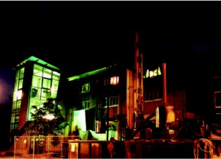
Drillmasters work day and night in order to get the coal mine gas out of abandoned mine shafts
