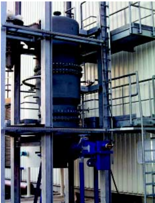
Fluidized bed plant for gasification or combustion of biomass feedstocks
