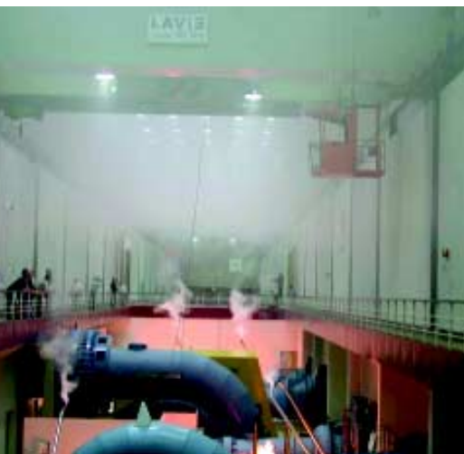
Hot smoke test in a machine cavern
