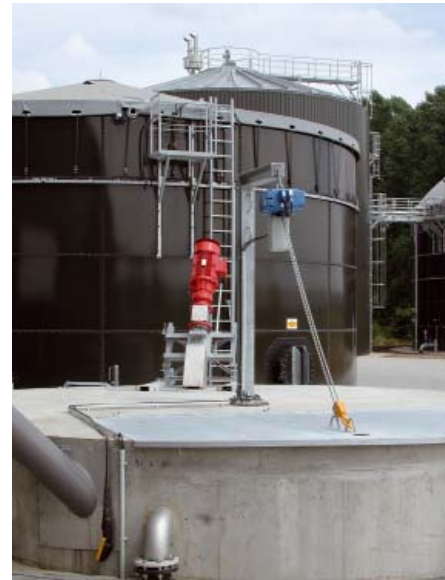
Biogas plant Schloss Wissen – View on the collection pond, buffer tank, and digester
